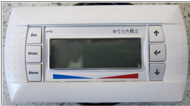
Fig. 4.1:pGD0 control panel
